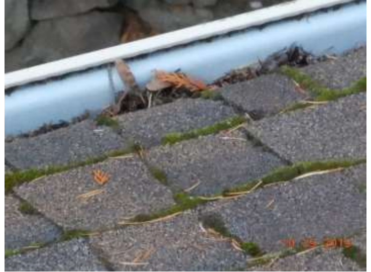
Moss on the roof
