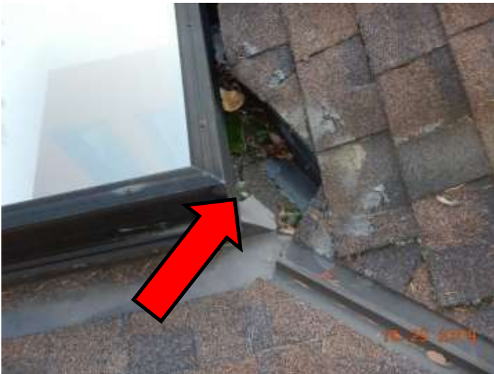
The area above the entryway skylight should be kept clean of debris
