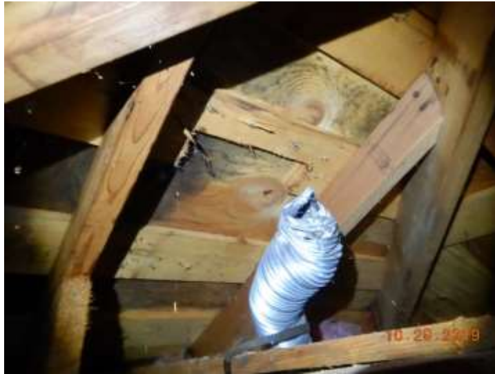
Bath fan ventilation duct does not extend to the exterior
