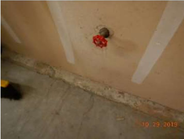
Domestic water shut off
