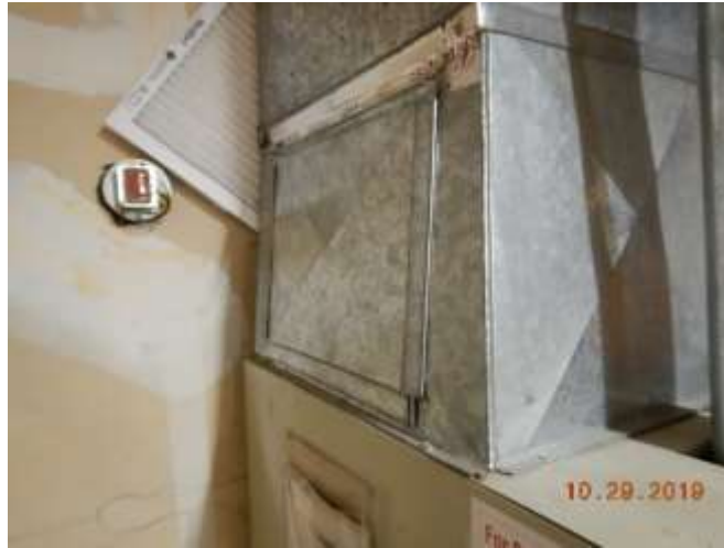
Furnace filter location
