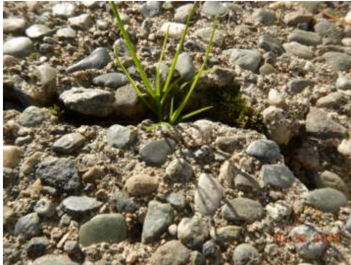
Cracks at the driveway
