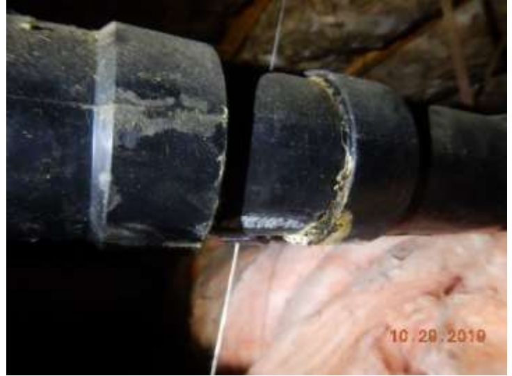
Leakage at the waste lines
