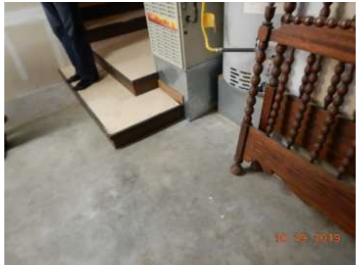
A vehicle can hit the furnace and water heater
