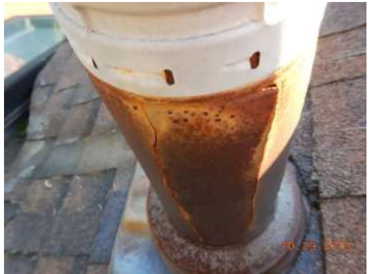
Detrioration of the furnace flue
