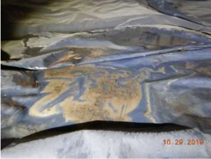
Waste water on top of the vapor barrier
