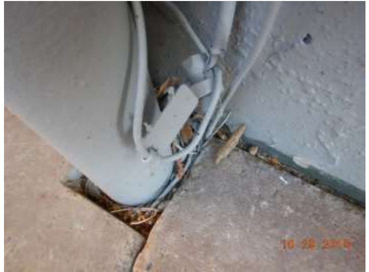
Electrical system grounding
