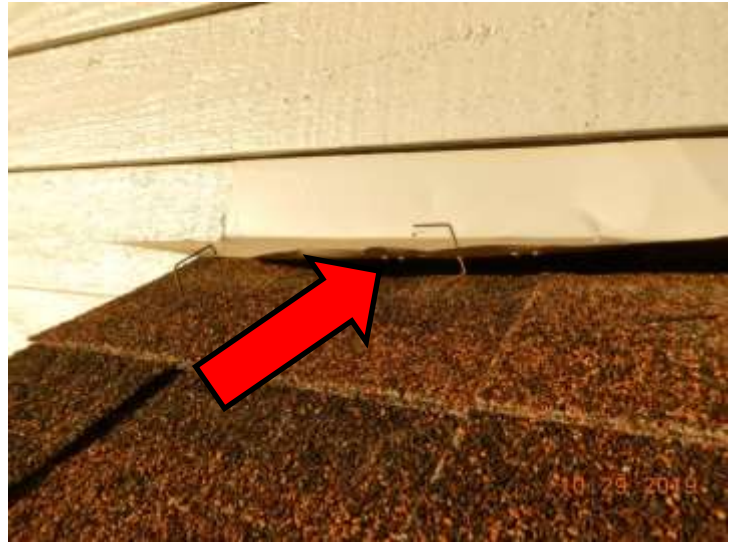
Loose roof to wall flashing
