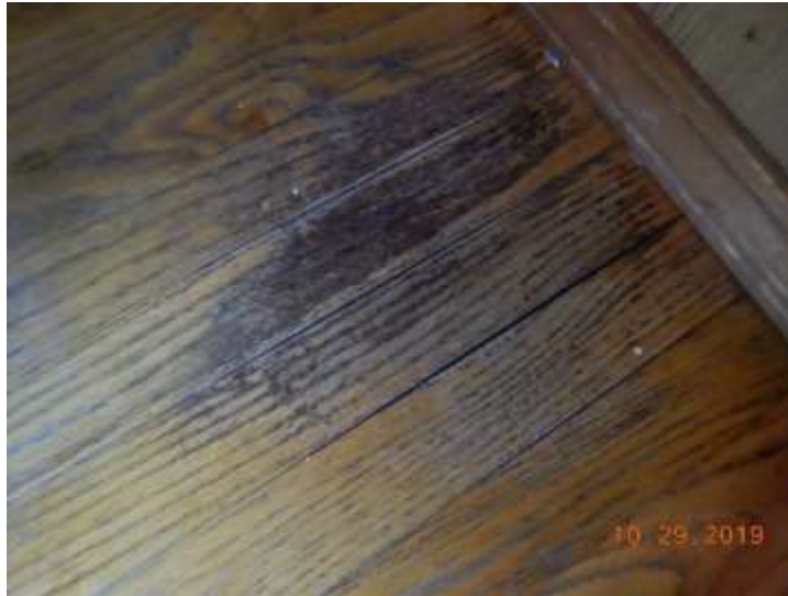
Moisture damaged hardwood floors; appears to be related to a dog water dish
