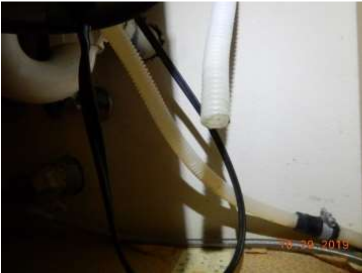
Dishwasher drain. The old air gap has been by passed
