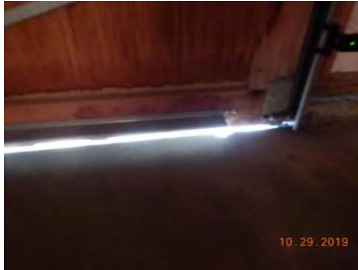
Gaps below the garage door
