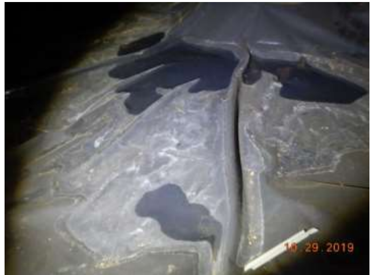
Puddles near the crawlspace access (below the waste lines)
