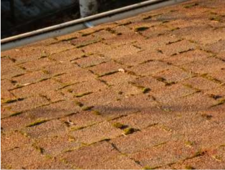
Moss on the roof
