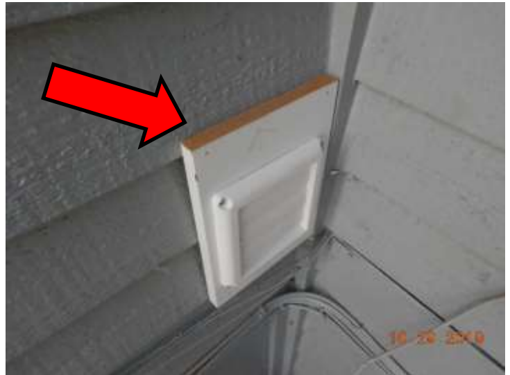
The block used at the dryer vent is not rated for exterior use. At a minimum, the top of the cut board should be painted
