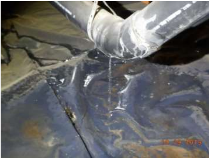
Leakage from the waste lines (approximately 10 feet from the front of the Living room)
