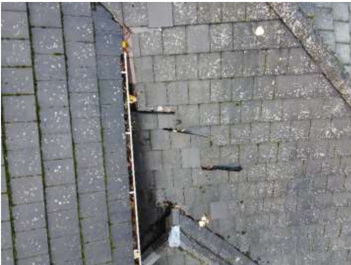
Diverter flashing is installed at the roof above the area of leakage at the S.E. corner of the Living room
